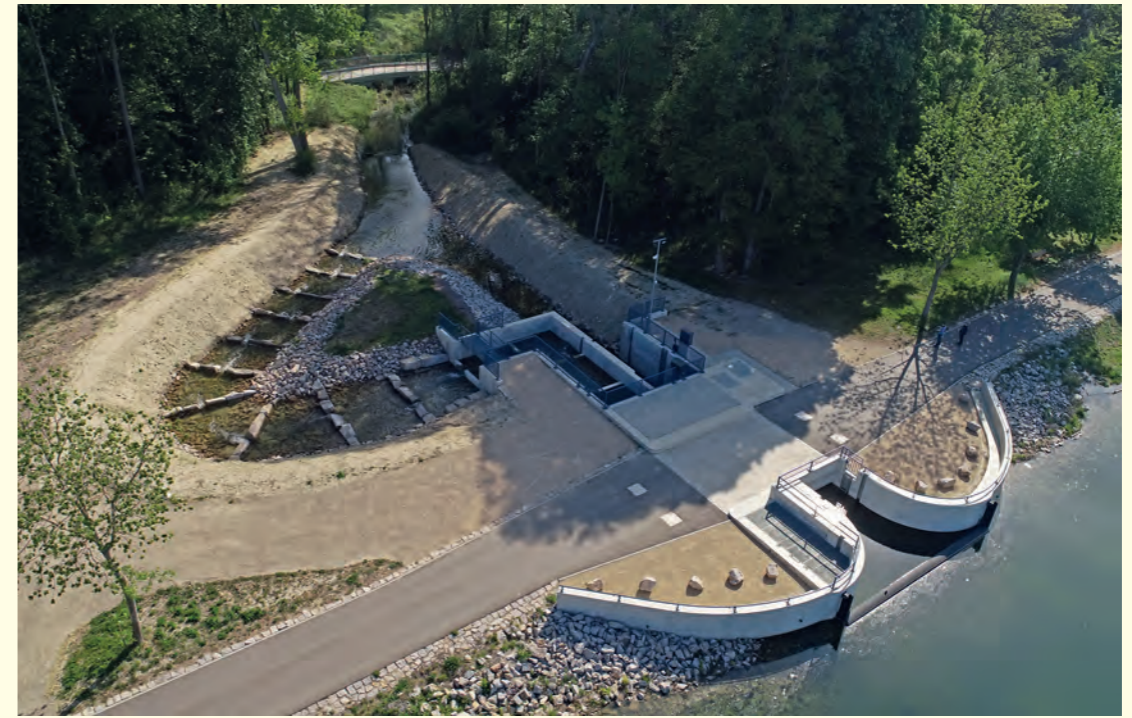
Ecology and technology working hand in hand: flood retention area at the Breisach irrigation barrage with inlet structure and fish ladder
